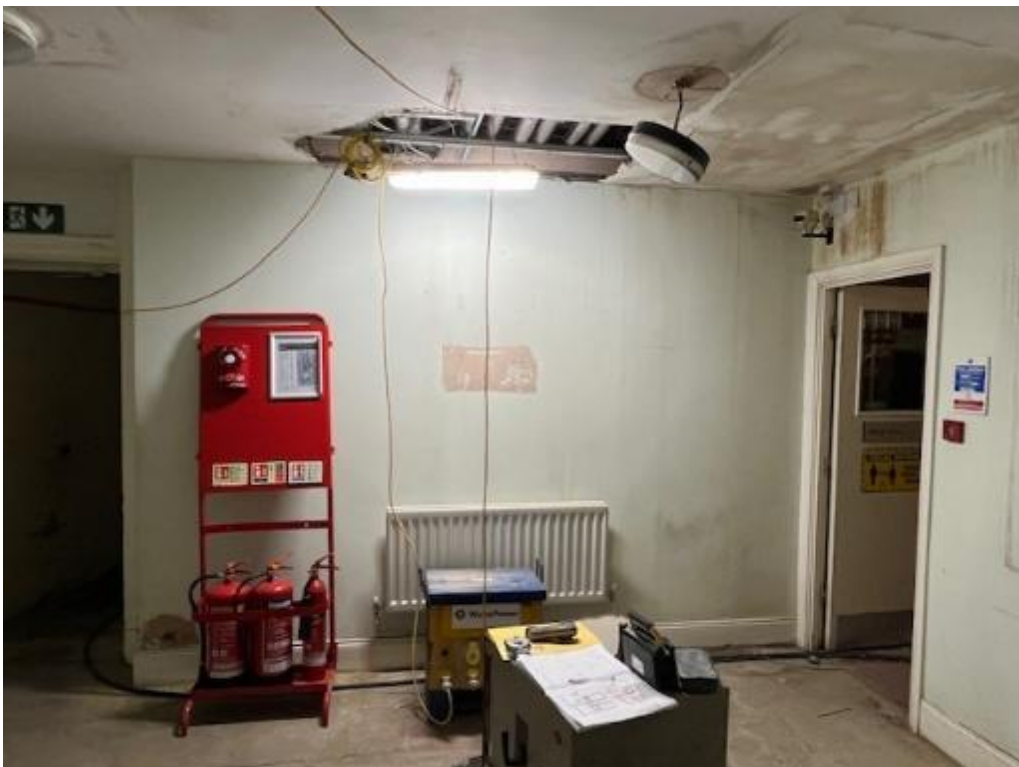
P61 – Chimney – drylined ( Note: damp staining)
