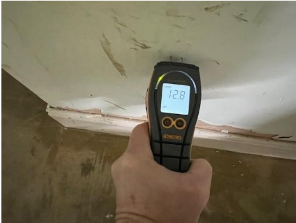
P64 – Wall 12.8% moisture content
