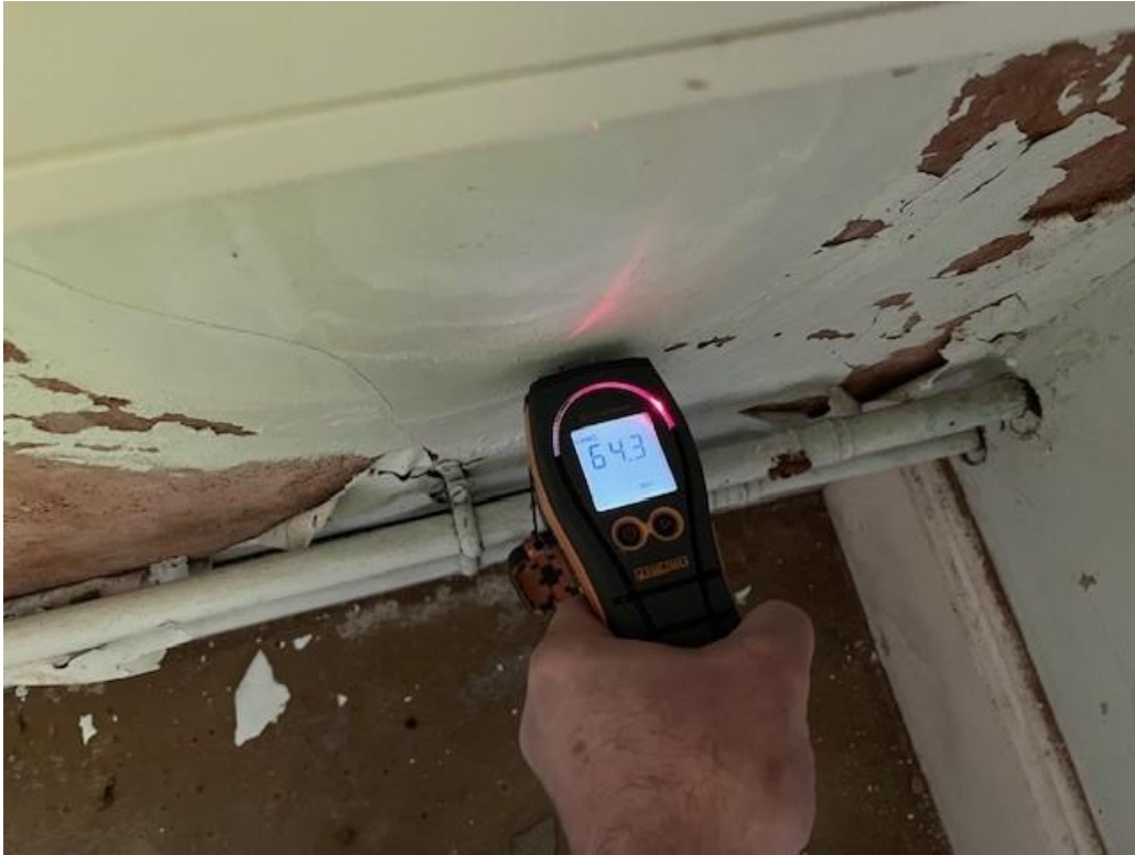
P45 – Director of Estates 64.3% m.c note damaged paintwork and plaster
