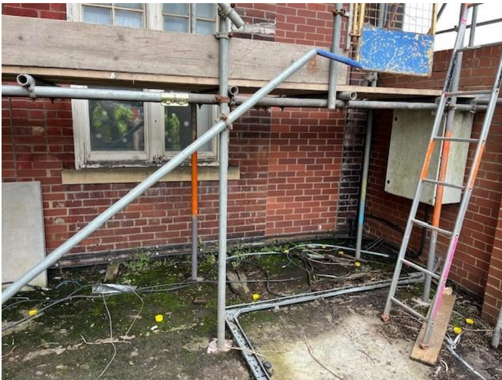
P36 – West Elevation yard – surface water ponding against the external wall of the building
