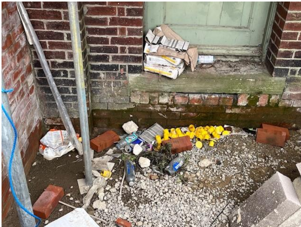
P22 – East Elevation brickwork below door threshold saturated
