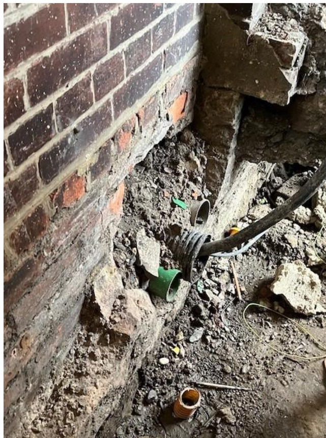
P9 – East Elevation services penetration below ground level Note ground level above finished floor level
