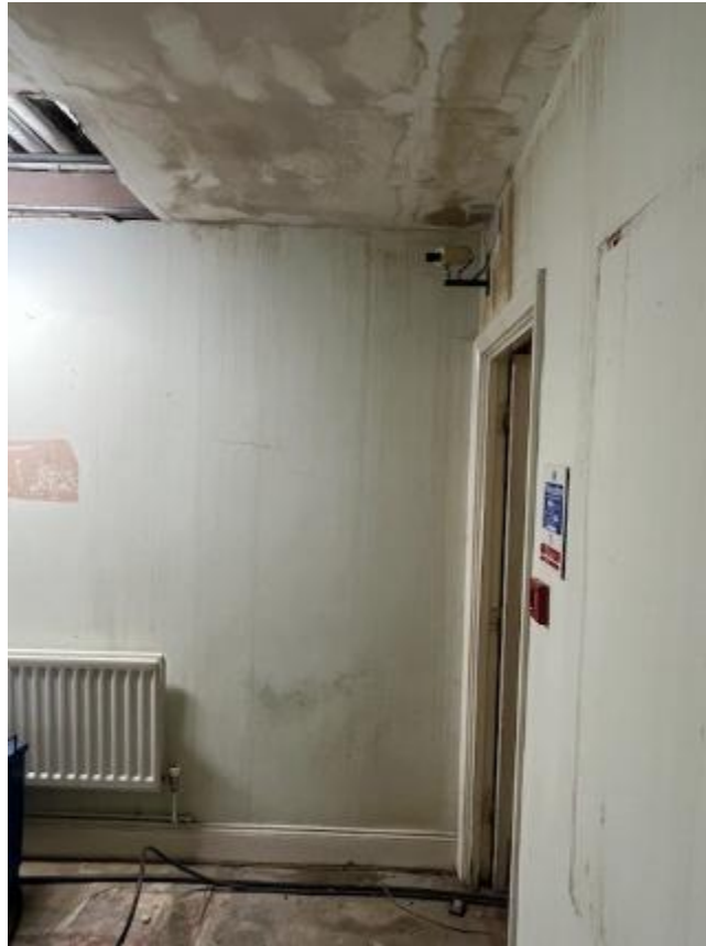
P62 – Chimney/adjacent ceiling penetrating dampness evident
