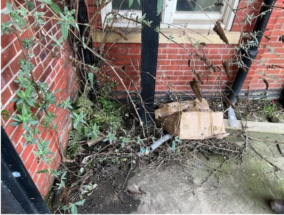
P47 – West Elevation – buddleia growth and blocked gulleys
