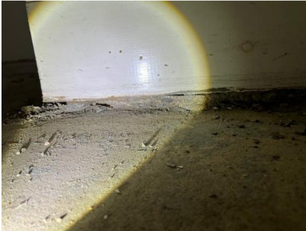
P74 – Potential bridging caused by migration of moisture via plaster in contact with the floor
