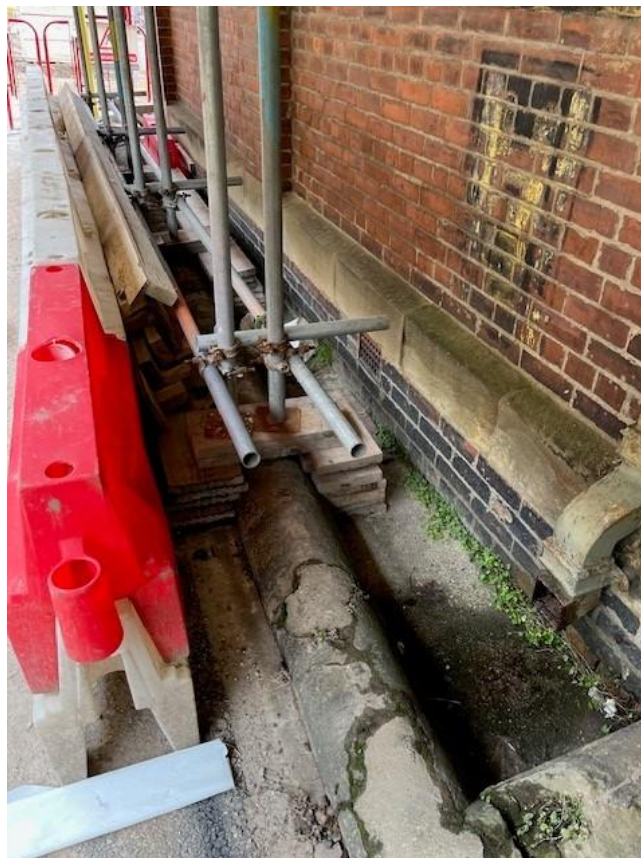
P56 – North Elevation rainwater pipes discharge onto solid concrete contained within a stone plinth course
