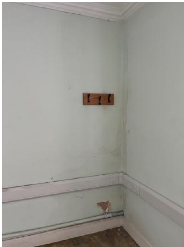
P38 – Visual evidence of penetrating dampness
