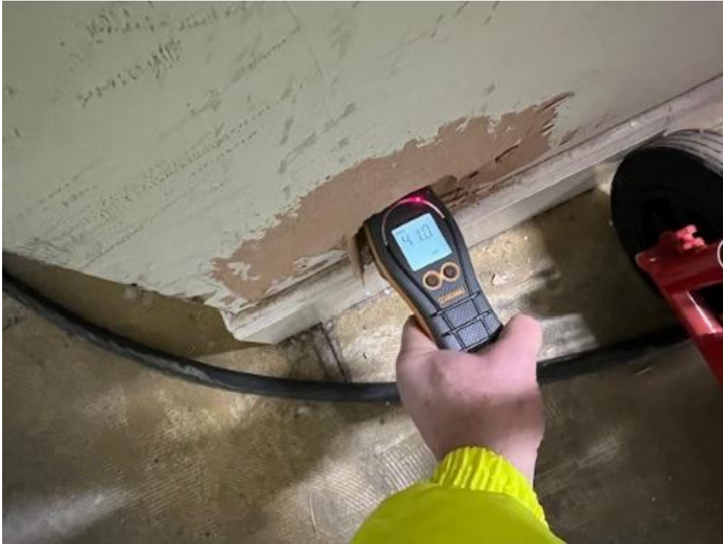
P60 – Chimney – 41% moisture content (concealed behind drylining)
