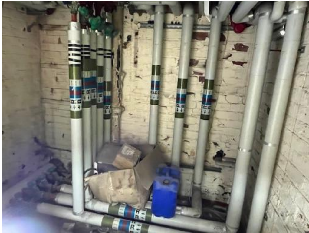
P57 – Plant Room penetrating dampness from front roof
