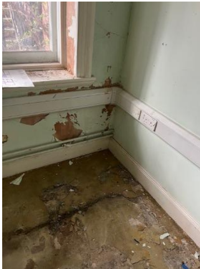
P46 – Visual evidence of flaking paintwork and damp plasterwork
