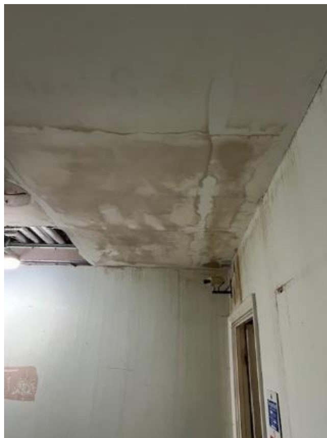
P52 – External wall and ceiling of Circulation Area 2 affected by roof leaks -penetrating dampness from failed rainwater pipes
