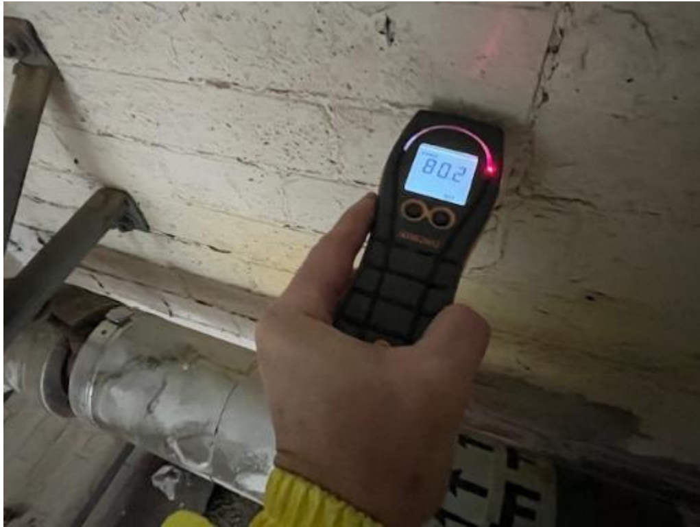
P59 – Plant Room 80% moisture content
