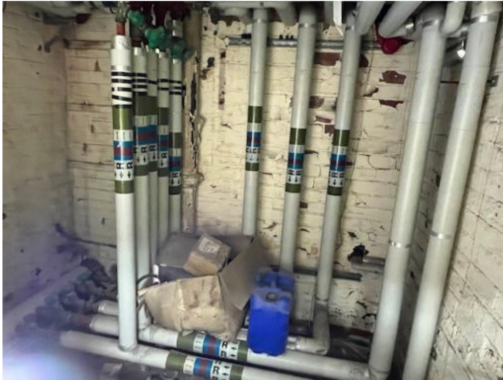
P53 – Plant and Storage Room 25.7% moisture content due to penetrating dampness
