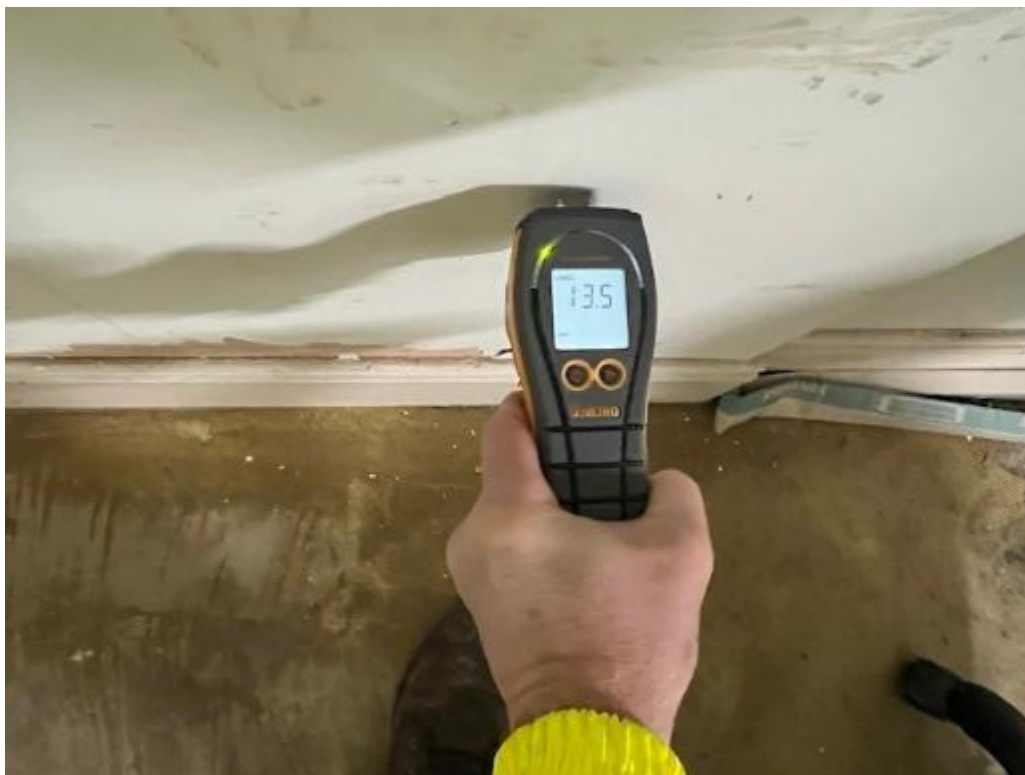
P65 – Wall 13.5% moisture content
